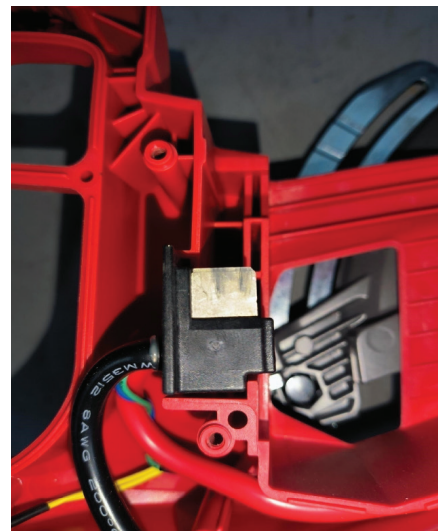
6) Closeup of Battery Terminal Block and wires.
